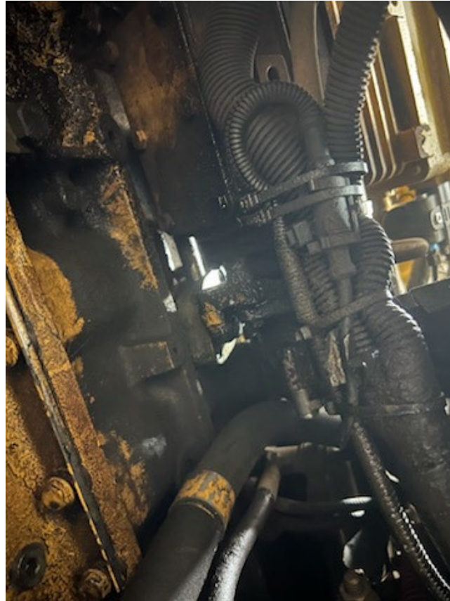
Power Steering Pump Leak
