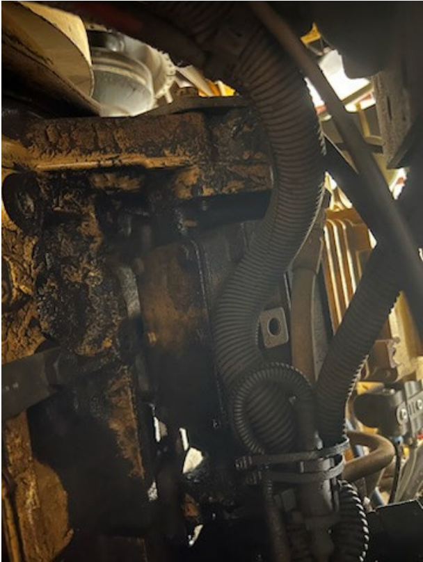
Air Compressor Oil Leak
