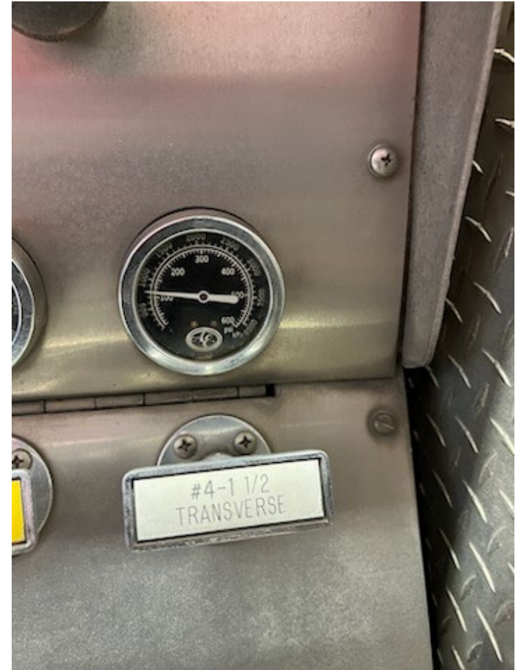
Bad Pump Panel Guage
