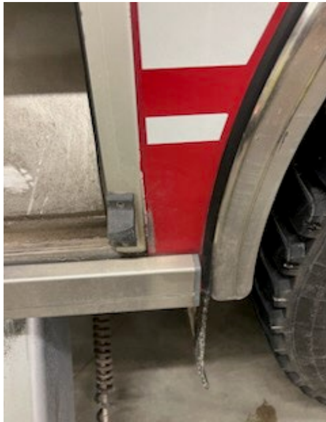
P1 Door Damage
